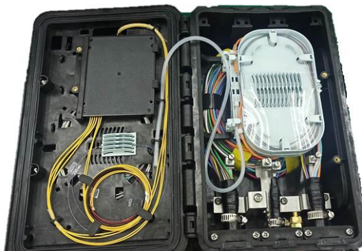
Input Port and Signal Port: Routed in Splice Tray for Feeder Cable Integration
